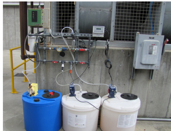
Automatic control system with double contained chemical Storage
